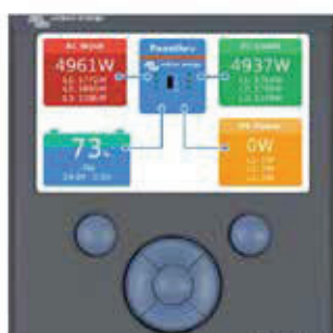
Color Control GX, showing a PV application
