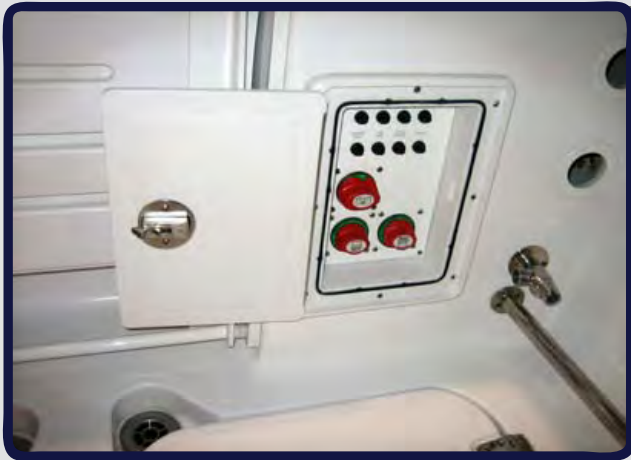
Battery Switch Electronics Panel Door with Poly Frame
